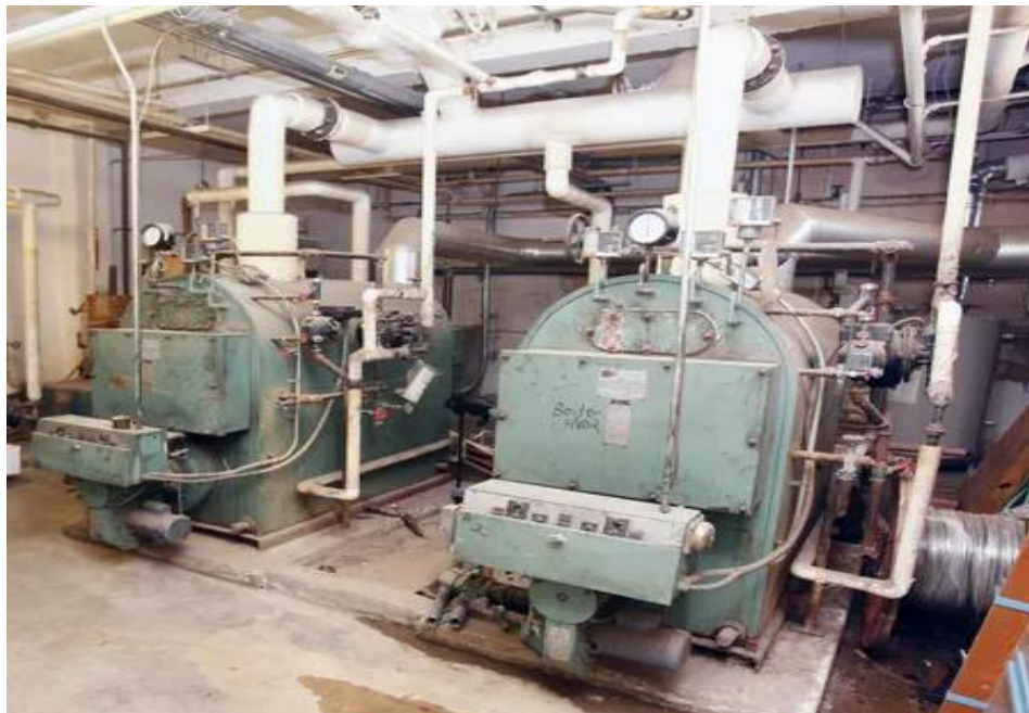
Less Efficient Boiler Systems
