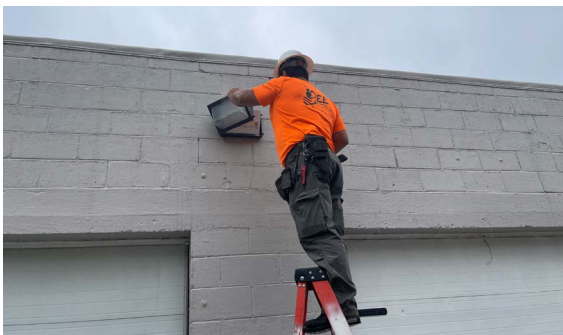
Gus Bautista (Bee Electric) updating exterior lighting
